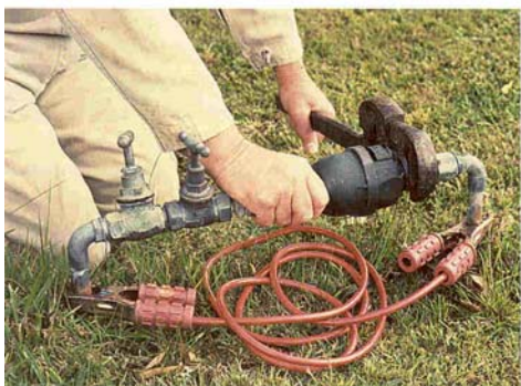
Remember to have bridging conductor in place when working on mains water supplies
