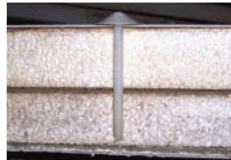
This photo shows the edge of one of the panels, with a broken nylon mushroom head bolt showing it broken near the surface of the panel
