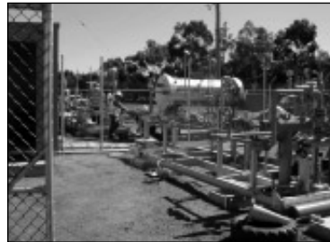
Longford Gas Metering Site
