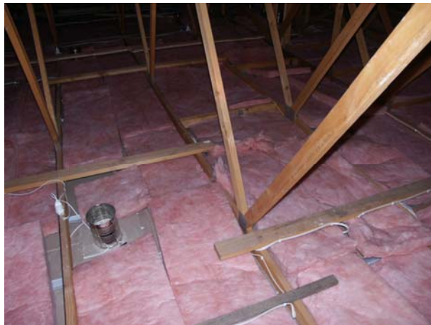
Poorly installed insulation
