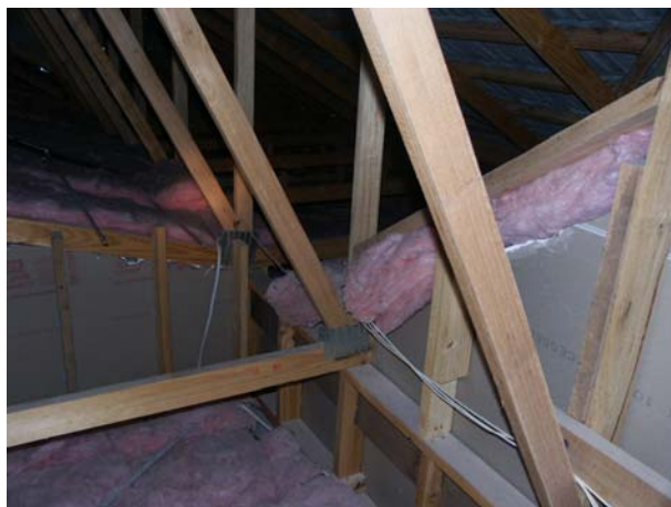
Insulation has not been included on vertical walls to fully insulate the ceiling space.
