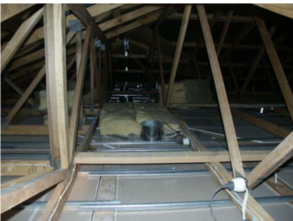
Insulation not installed.
