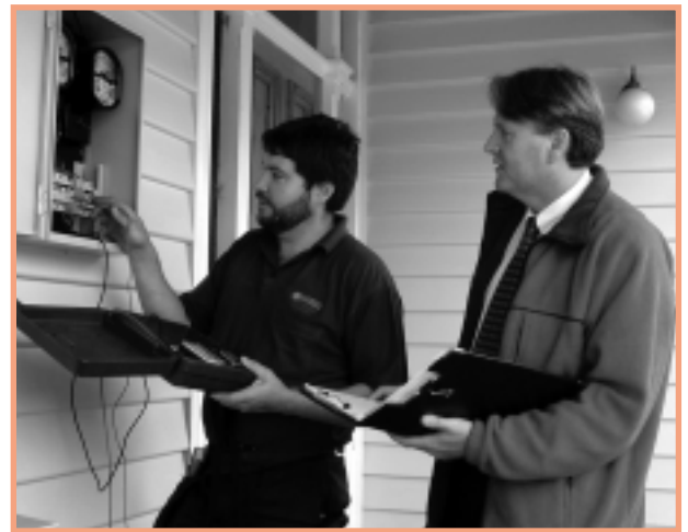
Electricity Safety Officer, Tony Millhouse and Earle Patman of Sackett Services participating in the installation testing audit.
